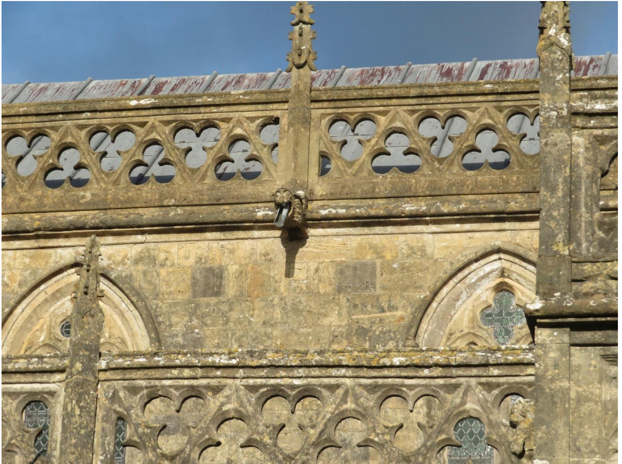
Fig 43: Gargoyle location below top parapet.
