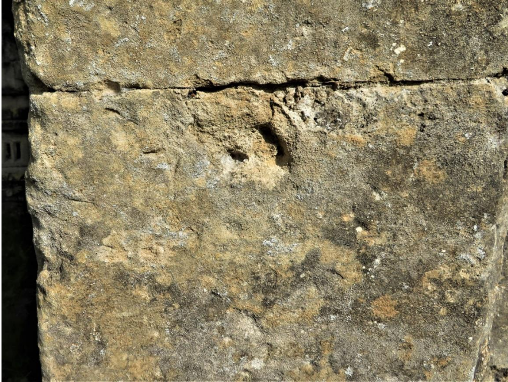
Fig 29: Circular feature left hand side of porch.
