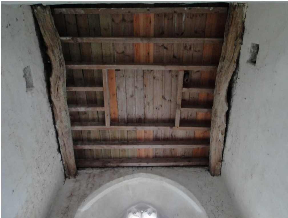
The ceiling incorporates beams (perhaps 18th century). Sockets in the walls below may indicate an earlier ceiling / belfry floor.
