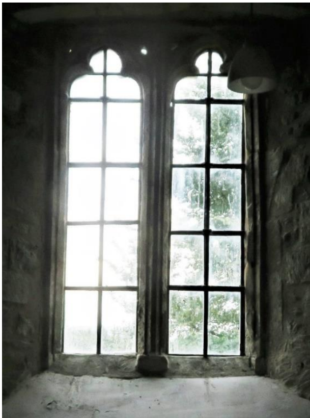
West of blocked door. A particularly splendid. 15 th or 16 th century window.
